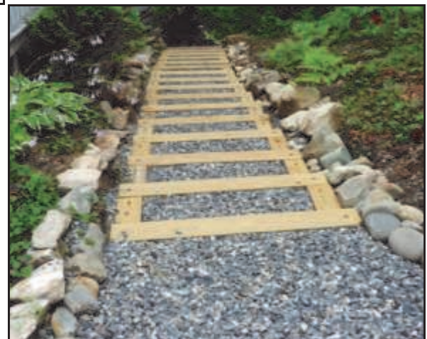
15 Infiltration Steps leading down to Long Pond. Top is before and bottom is after the project.
